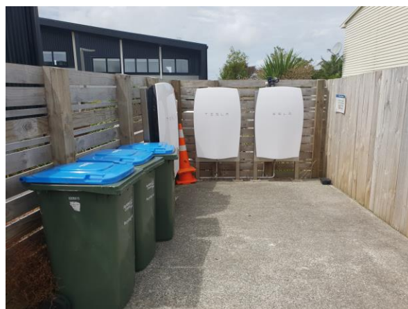
Figure 7: The development was the first to include Tesla power batteries, where energy produced from solar panels on the roof is stored and distributed to households.
